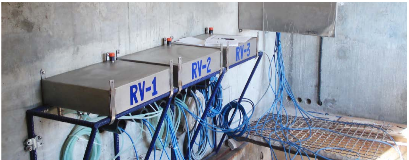
Reference vessels in Sogamoso HPP project, Colombia
