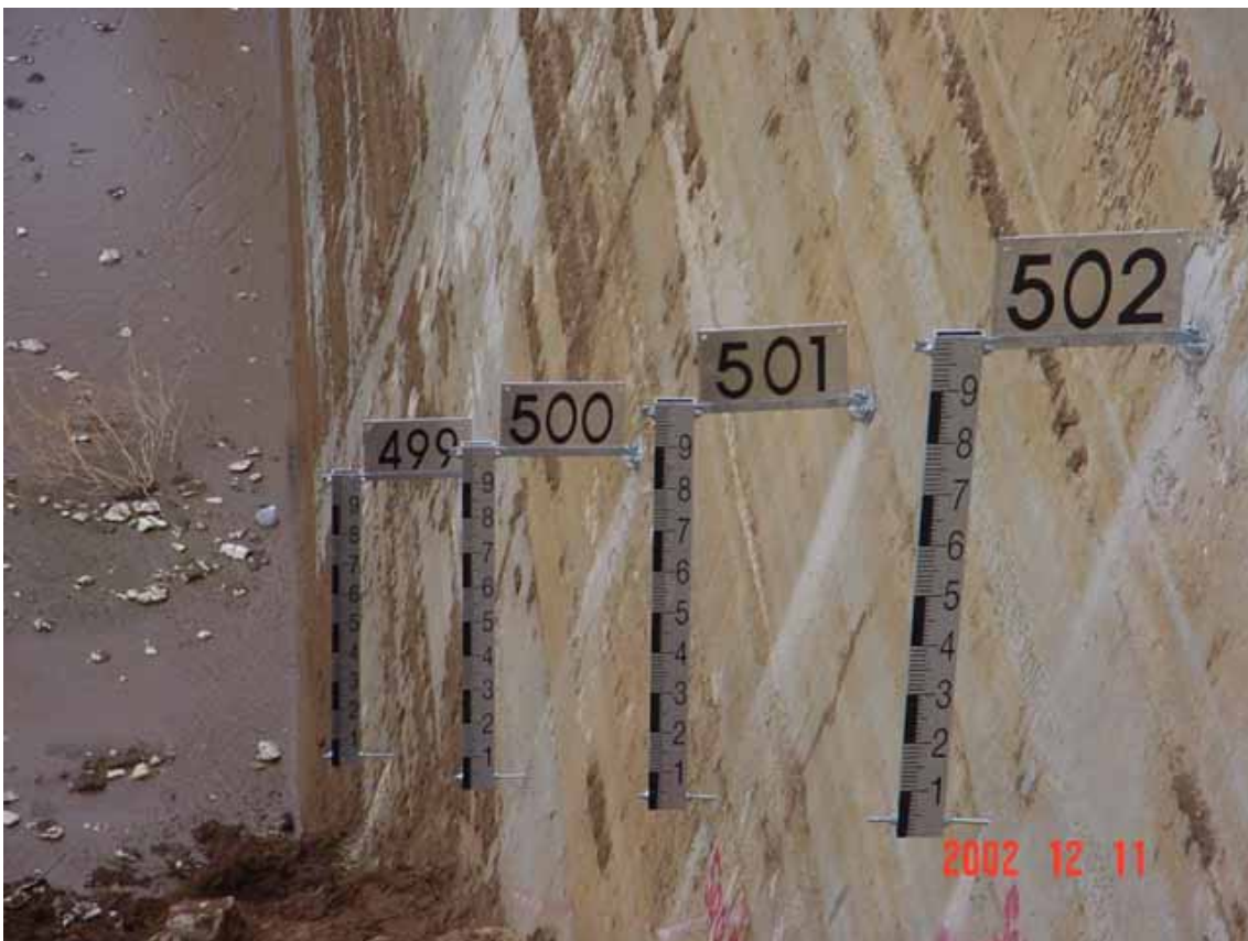
Staff gauges for direct reading of basin level
