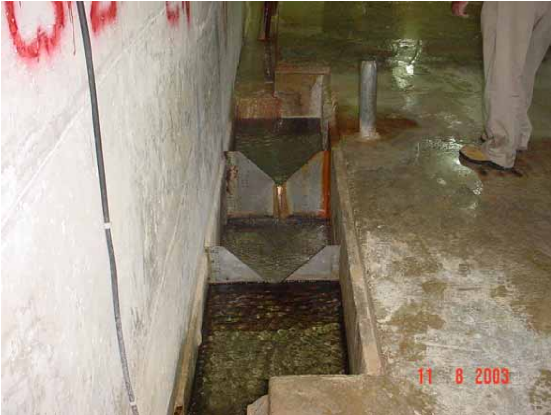
V-notch weirs for leakage measurement
